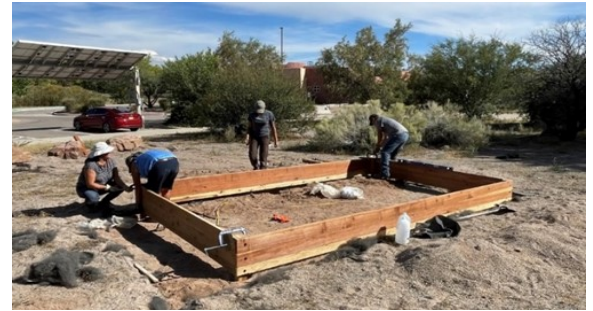
Figure 1. Students and faculty of the Advanced Technical Education (ATE) Department installing the new SIPI FarmBot system near the Science and Technology Building
